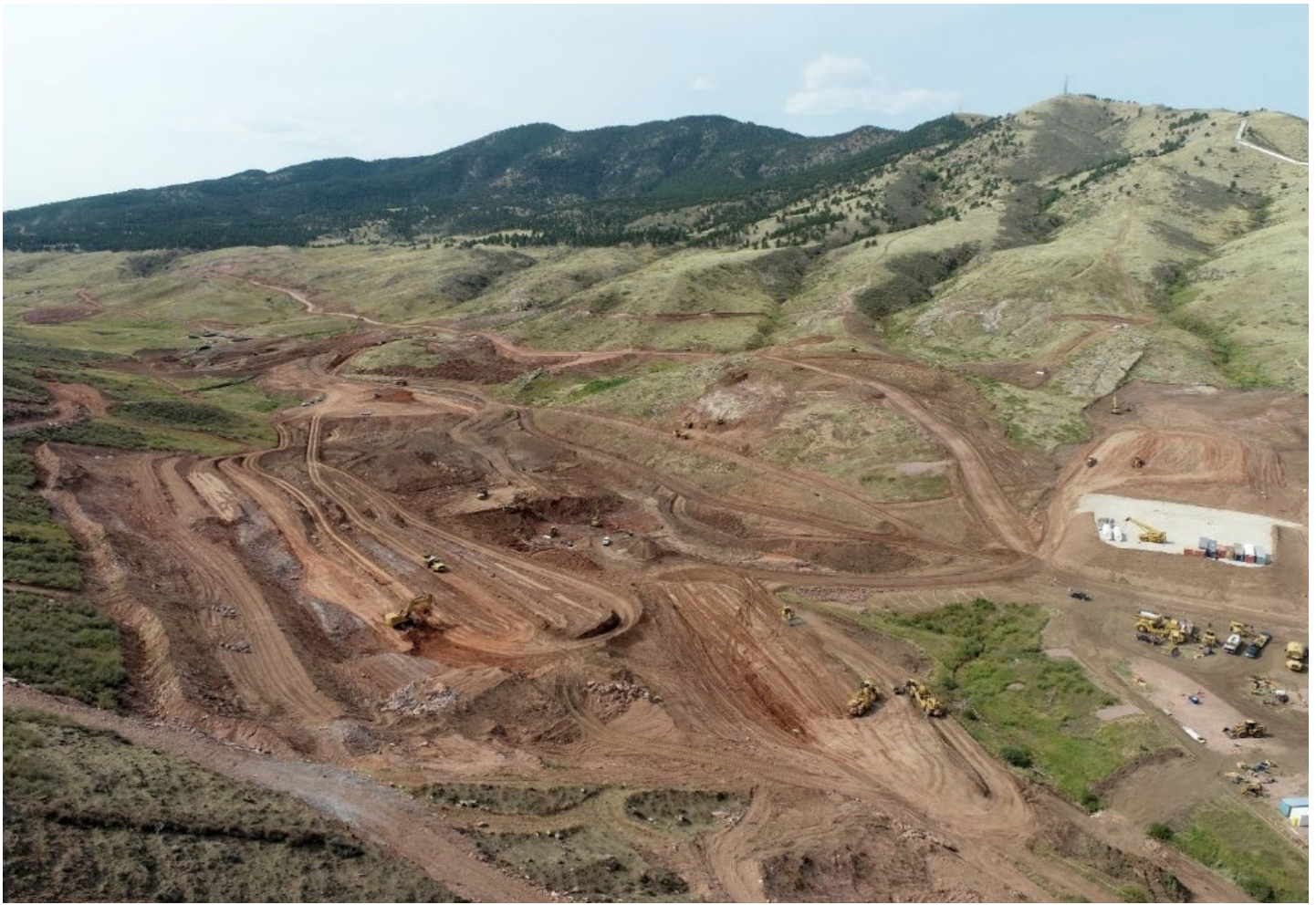
An aerial overview of construction on the Chimney Hollow Reservoir Project on September 30, 2021.
