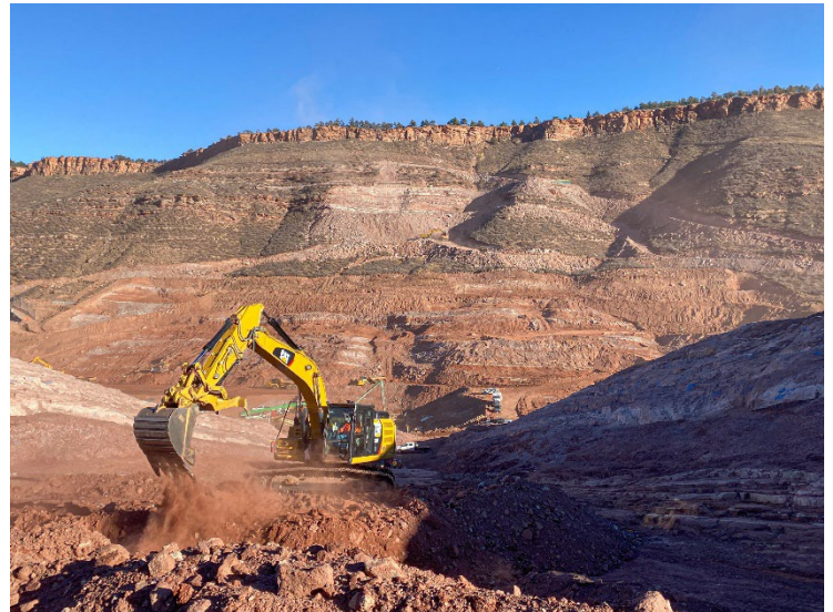
Work on the main dam at Chimney Hollow Reservoir Project here and below.
