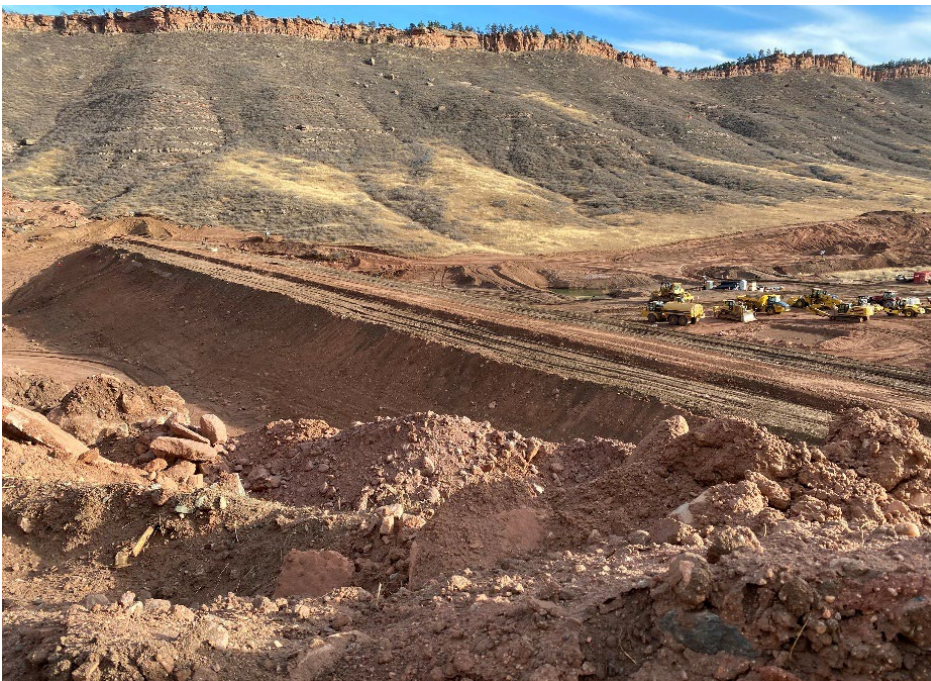
Construction of the cofferdam at the Chimney Hollow Reservoir Project underway in late 2021.
