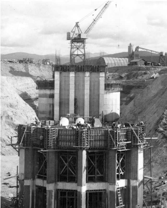
Crews construct the inlet structure on the Granby Pump Plant, later renamed Farr Pump Plant, in September 1948.
