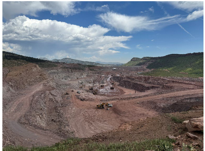
The on-site quarry produces all the rockfill for the main and saddle dams.
