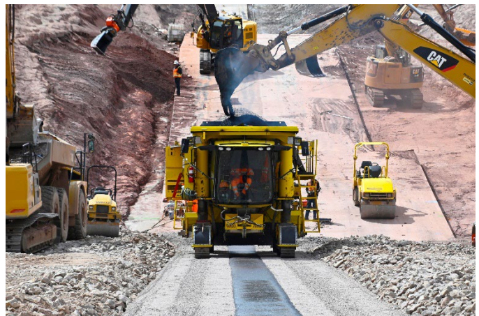
The paver laying down the asphalt core on the main dam at Chimney Hollow Reservoir.
